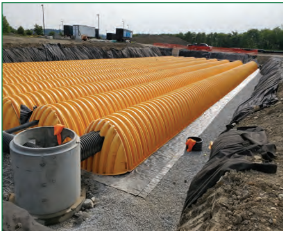
Photo shown above: MC-4500 ADS Storm Tech chambers installation (8 rows, 200 feet long and approximately 60,000 cubic feet of storage).
