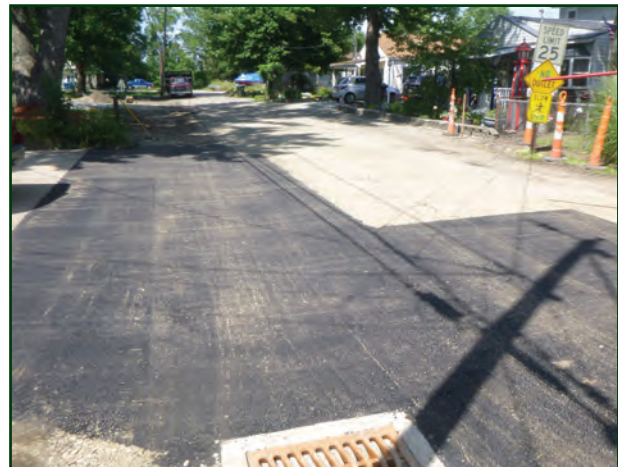
Photo shown above: New storm sewer on Lakeview Drive in the Village of Lakemore
