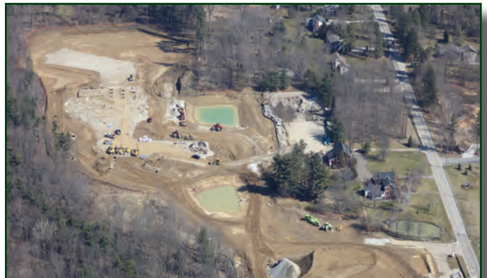
Photo shown above: Aerial view of Hudson Meadows Retirement Community under construction, (Courtesy of Cameron General Contractors)
